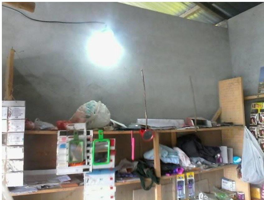
Figure 6: Solar light fixtures at homes of beneficiaries
