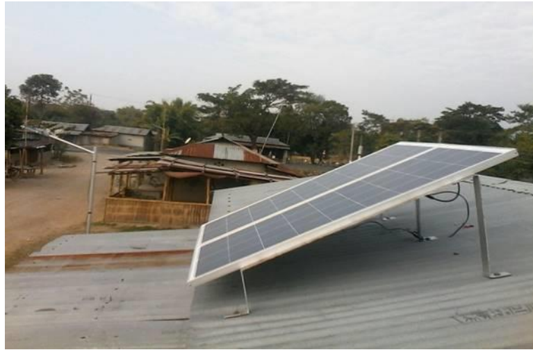
Figure 3: Solar PV Modules
