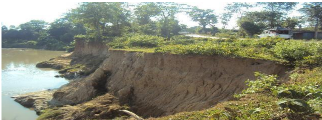
Teliamura-Khowai State Highway occupied by the River Khowai at Purba Kalyanpur
